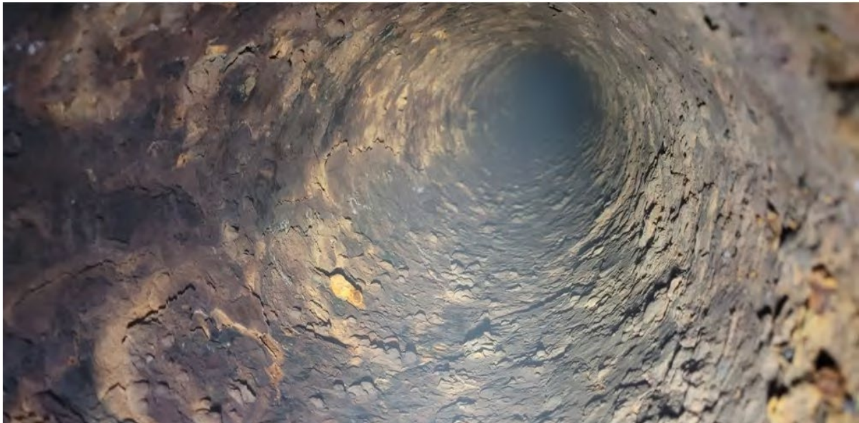
Figure 1. Condition of small diameter embedded pipe before surface preparation.
