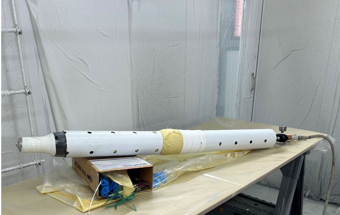
Figure 4. Pipe packer inserted into a pipe with holes and a break between pipe sections. The FRP repair is wrapped around the pipe packer, inserted into the pipe, and inflated to press the repair against the host pipe.
