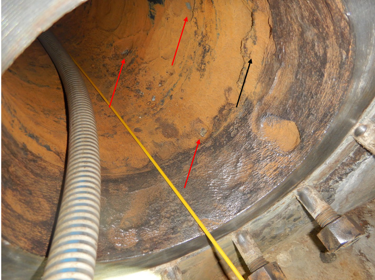
Figure 2. Condition of the small diameter embedded pipe after waterjet cleaning. Exfoliated iron oxide (black arrow) can be seen that wasn't removed by waterjet cleaning, as well as occasionally concrete is exposed (red arrows).
